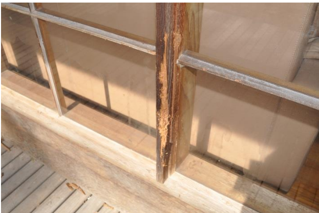
Figure 5: Cockatoo damage to timber window frames
